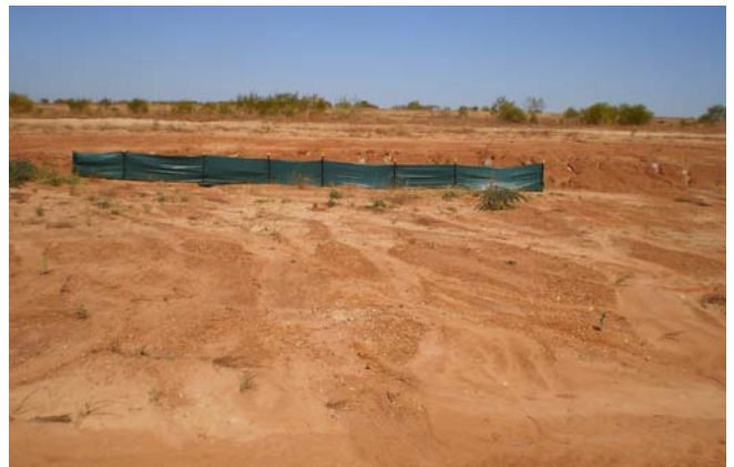
TSF Cell 1 Cap with mesh fence to stop erosion. The cap needs to be shaped next audit.
